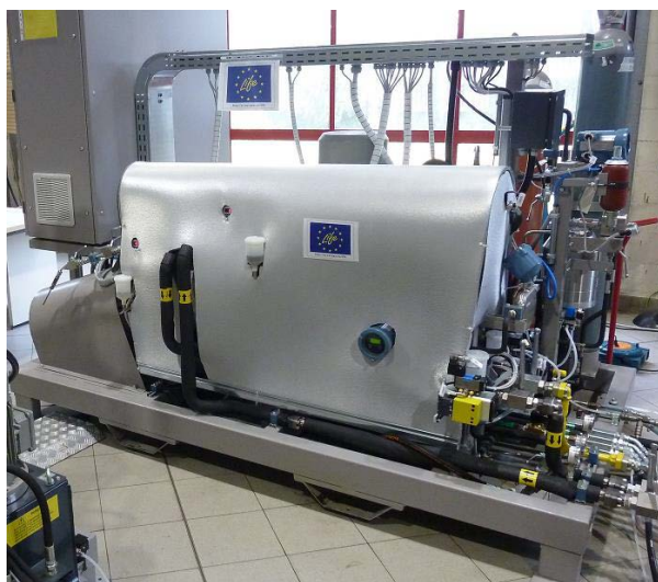
Figure 3: Part of k12 pilot plant at Afros facility
